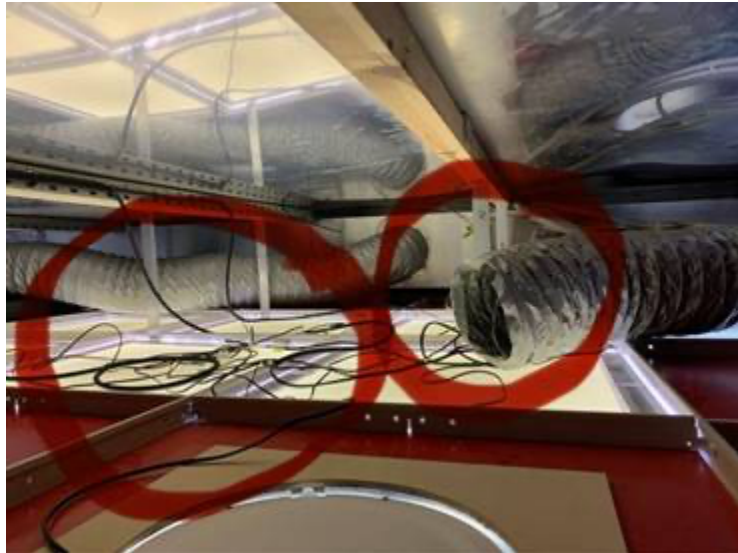
Figure 20. Loose cables trailing on the suspended ceiling within the RF cage are known to be a source of RF spikes and should be avoided by use of secure cable trays and mounting brackets.
