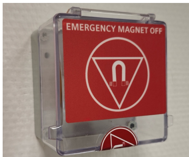
Figure 12. Example of wall mounted emergency magnet off button with protective guard flap to avoid accidental activation and the new signage label introduced in IEC 60601-2-33 (2022).
