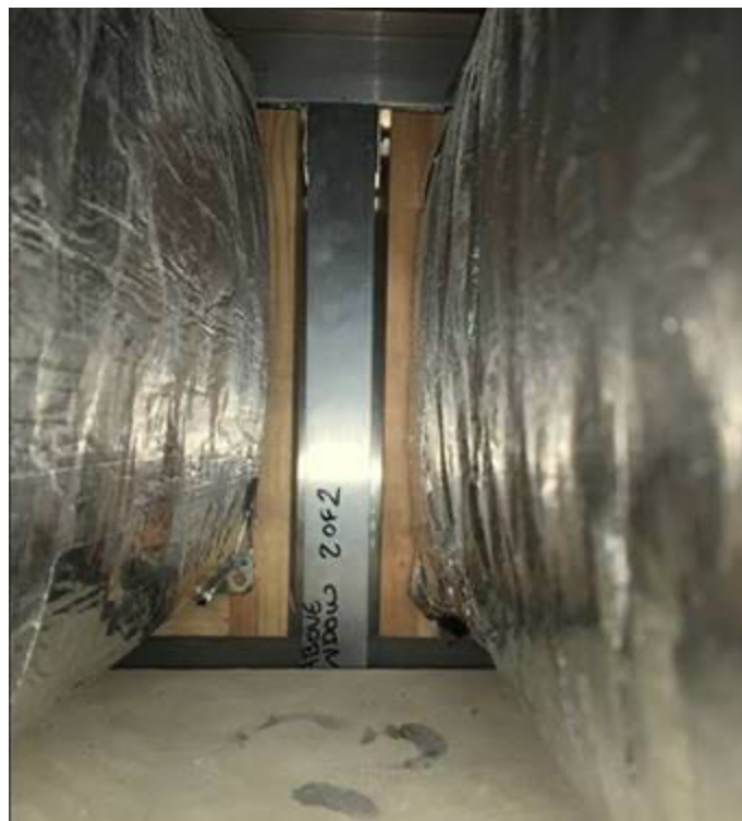
Figure 7. Example of wooden frame providing electrical isolation between honeycomb waveguides in the RF cage and external air ducting.
