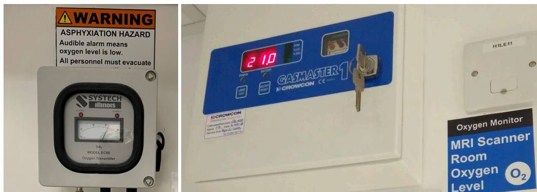
Figure 13. Examples of oxygen monitoring displays in the MR Control Room.
