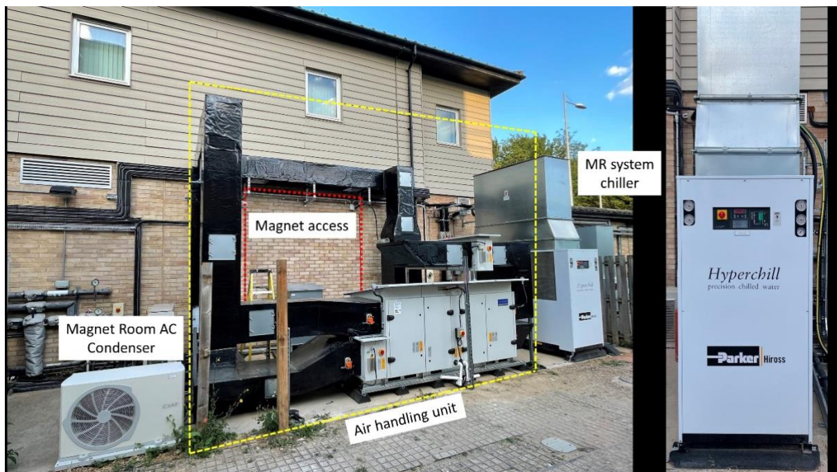
Figure 18. Example of MRI supporting plant. The air handling unit is highlighted by the yellow dotted box. Also shown is the condenser unit for the MR Examination room air conditioning and the MR chiller system that provides chilled water to the MR system heat exchanger located in the equipment room. The red dotted line partially shows the magnet access. This wall is demolished for installation/removal of the magnet.
